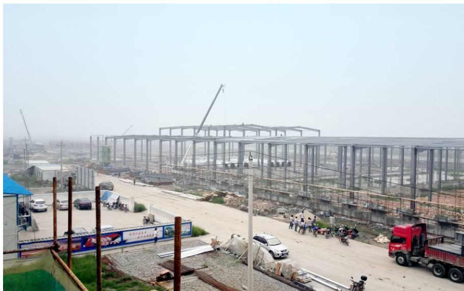
Full view of the construction work of Anhui Conch New Building Materials Company
