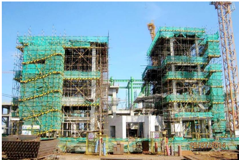
Full view of the Thailand SCG cement project raw material mill under construction in Indonesia
